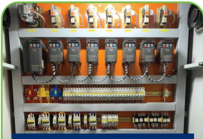
Multi Drive System Panel
