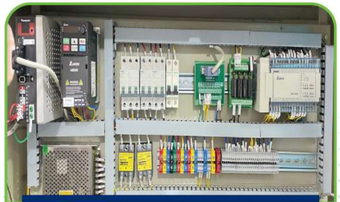
PLC, HMI automation Panel
